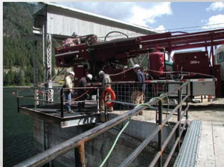
PPL Montana engineers and contractors work on the intake structure at Hebgen Dam.
